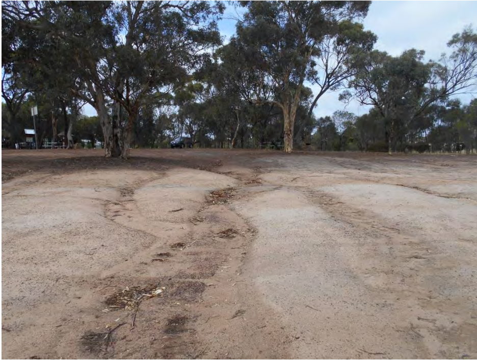
Plate 6: Erosion of banks of Railway Dam
