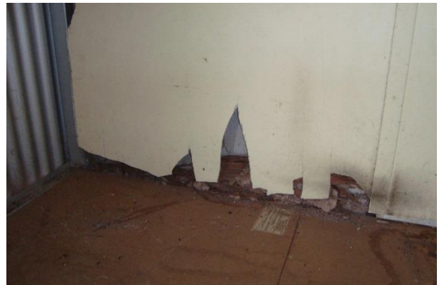
Internal club rooms white ant/asbestos damage
