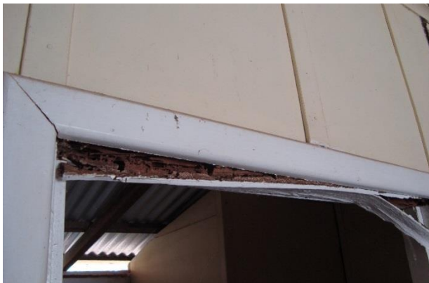
Internal Club rooms white ant damage
