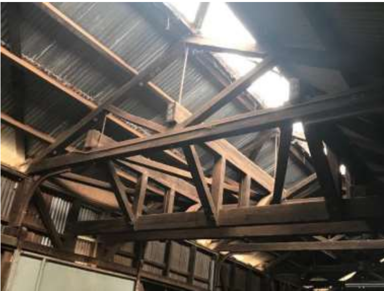
Photos 112-114 Goods Shed . Interior. View looking south along the east wall showing the remnant railway line; Views of the roof structure.
