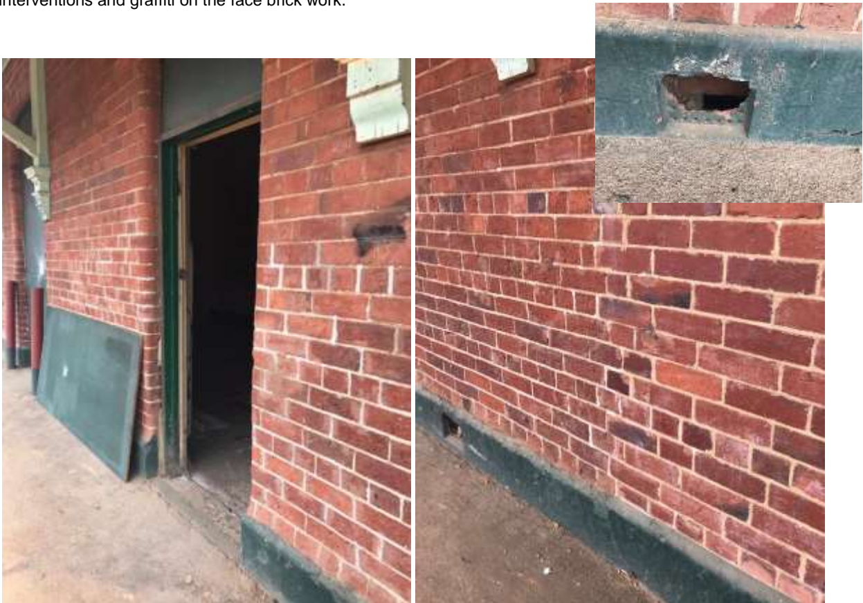
Photos 15,16 Narrogin Railway Station Details of parts of the east wall showing interventions in stretcher bond against the original brickwork in Colonial bond ( one course of headers and three courses of stretcher bond. Also note the bullnose bricks on the corners and doorways. Inset: damaged wall vents.
