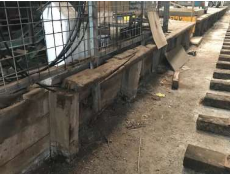
Photos 147-149 Goods Shed. Interior. The remnant railway on the east side (looking north); and the metal-framed storage area at the south end of the shed.
