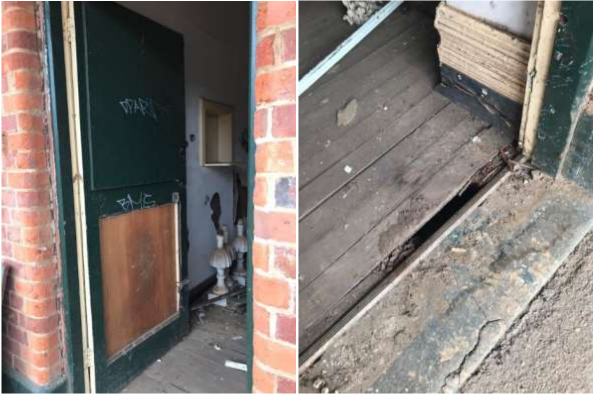
Photos 17,18 Narrogin Railway Station Entry into the second room along the east of the station, showing damaged door and threshold.
