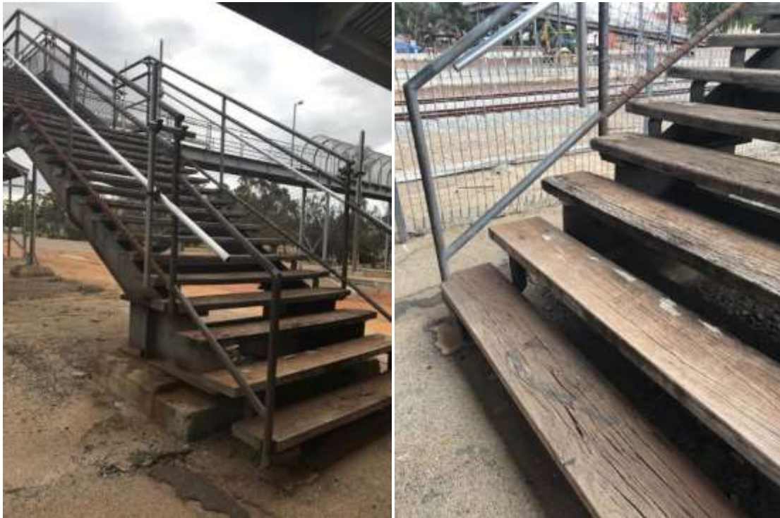
Photos 81-86 Narrogin Railway Station Pedestrian overpass: over Pioneer Drive to east; view south; steel structure with timber decking (83,84); and, timber stairs to access the railway station platform.
