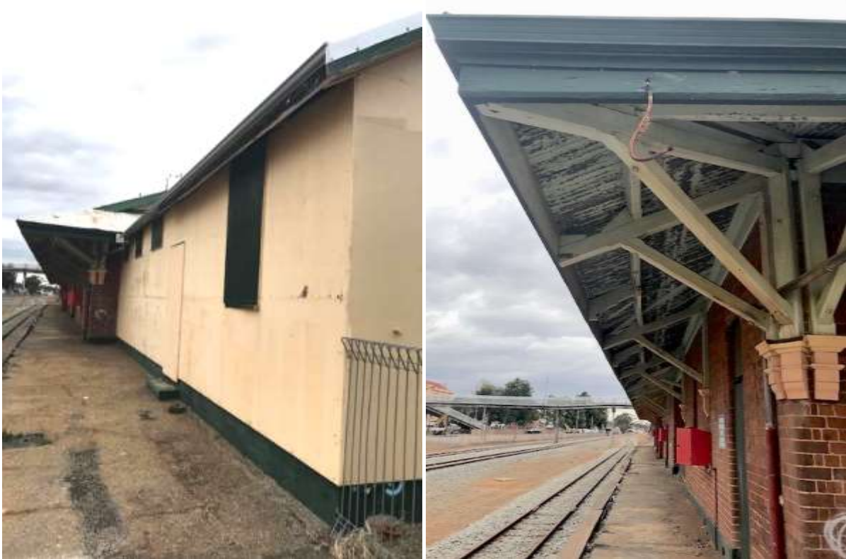
Photos 25, 26 Narrogin Railway Station Views looking north along the west platform showing platform damage.
