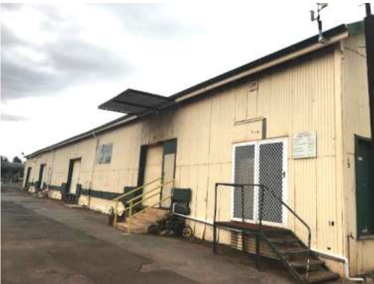
Photos 96-99 Goods Shed. Details on the west wall showing plumbing interventions, doorway and steps in one of the loading docks, and doors and stairs in the wall at the south end of the west wall.
