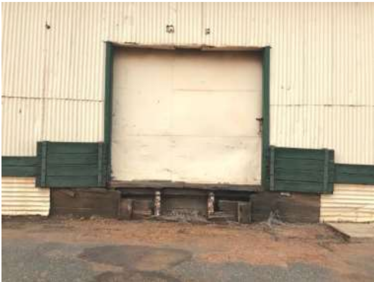
Photos 90-92 Goods Shed. View of the west wall showing the loading docks, condition, and interventions.
