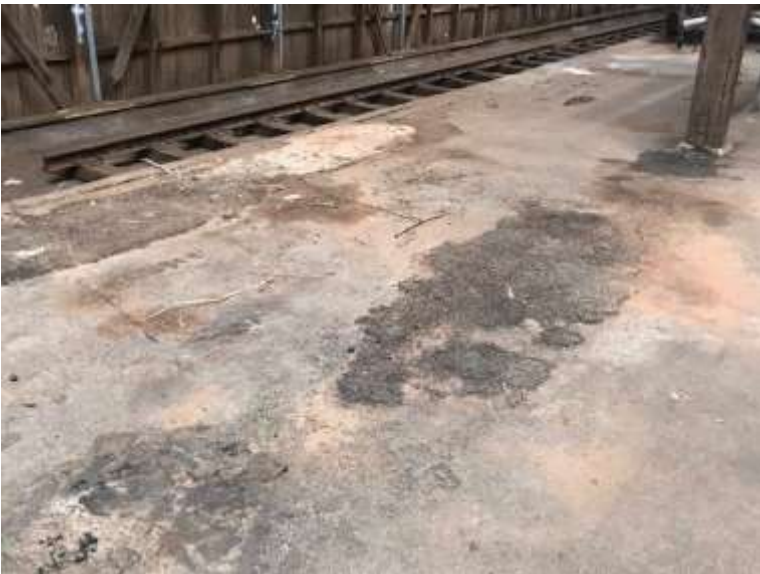
Photos 123-125 Goods Shed . Interior. Platform damage along the edge of the west wall and throughout the shed,
