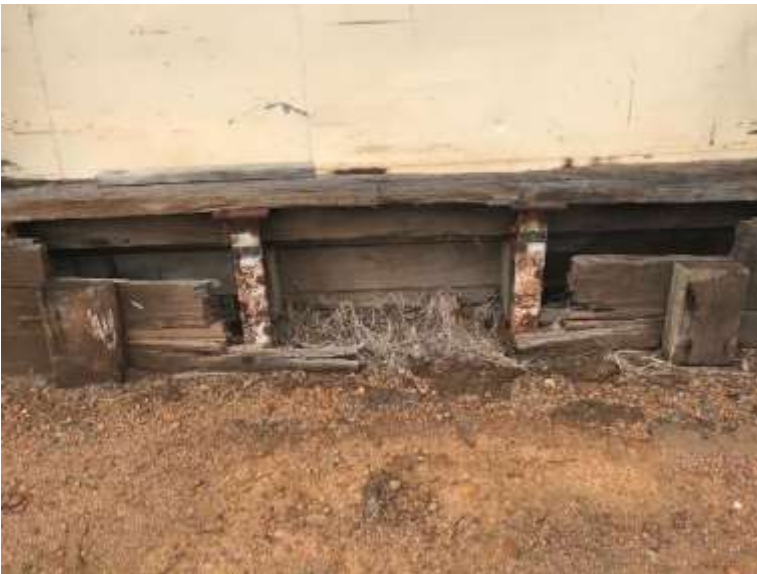
Photos 93-95 Goods Shed . Details on the west wall showing the loading docks, condition, and interventions.
