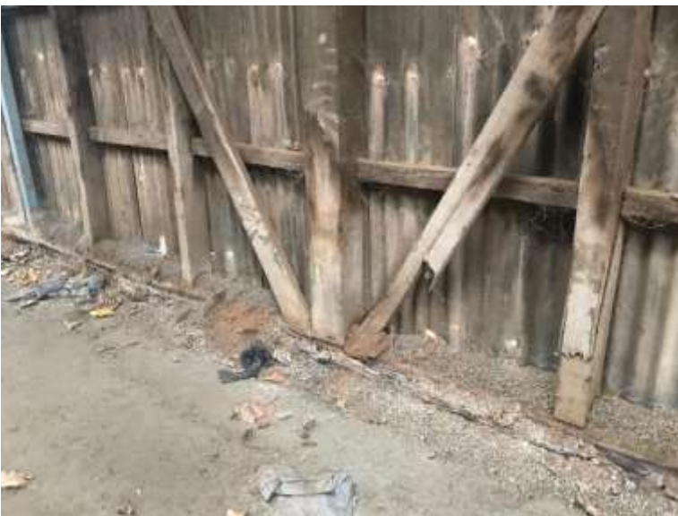
Photos 132-135 Goods Shed . Interior. The platform upstand and damaged edge; and, east wall structure damage.
